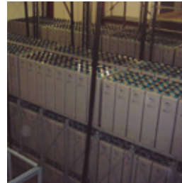
Colt Telecom in Amsterdam 24 OPzV 3000
