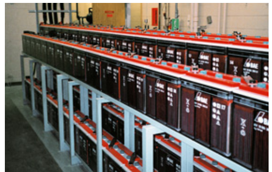
UPS application in USA 6 V 11 OGi 275
