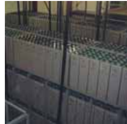
Colt Telecom in Amsterdam 24 OPzV 3000
